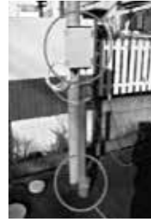
Fig 2. Example of a Water Level Sensor The device at the bottom is the water level sensor and the box at the top is the control box.
